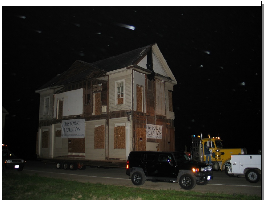
Missouri City law enforcement routed traffic around Highway 6 for the move so the whole convoy had good conditions to move the Dew House to Kitty Hollow Park.
